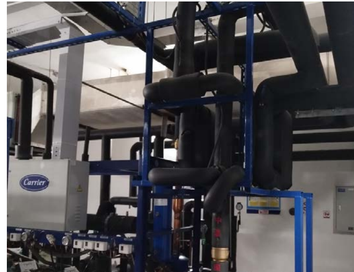
Plate heat exchanger
