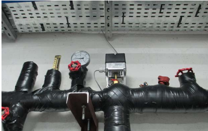
Three-way valve control of water and power
